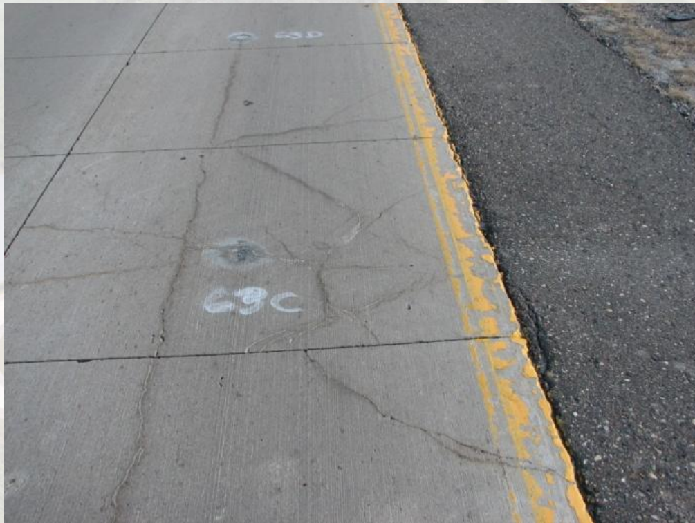
Figure 3. Cracked and “shattered” panels in Cell 63 (Fall 2010).
